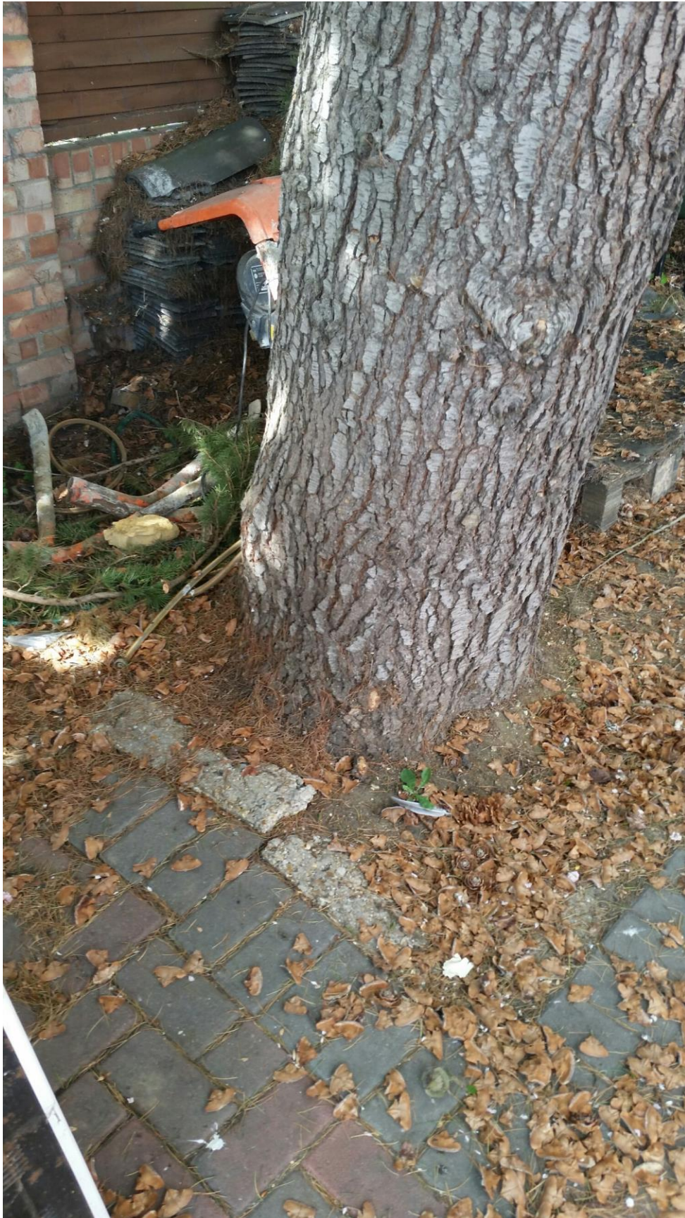
View of the base of T2 showing the extent of damage to driveway observed during site visit - taken 26 th April 2017.
